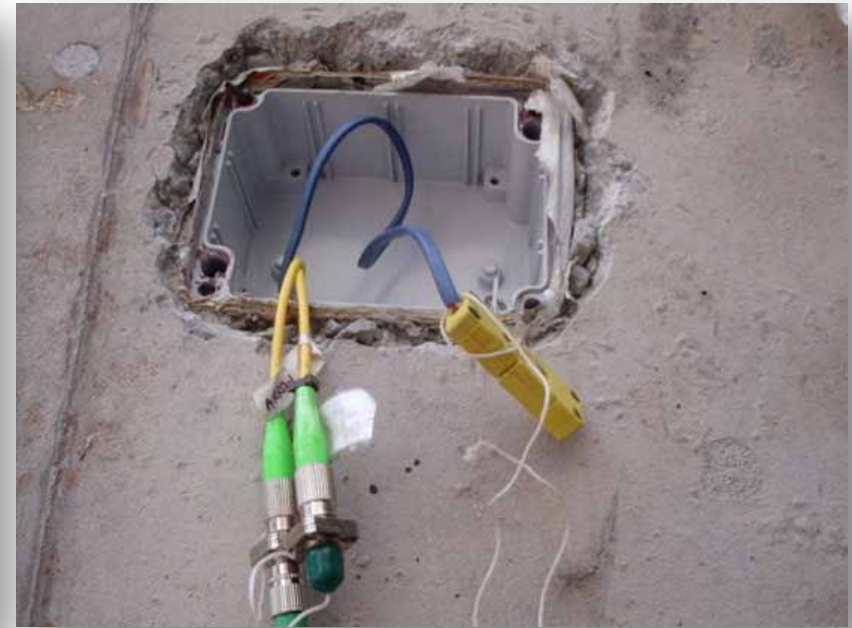
SmartBar Sensor cables exiting pillar.
