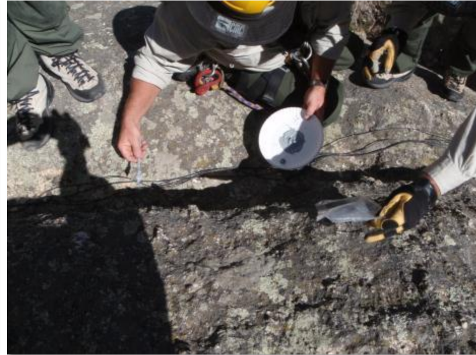
Securing the tie down clips to the rock with epoxy for securing the fiber cable runs.
