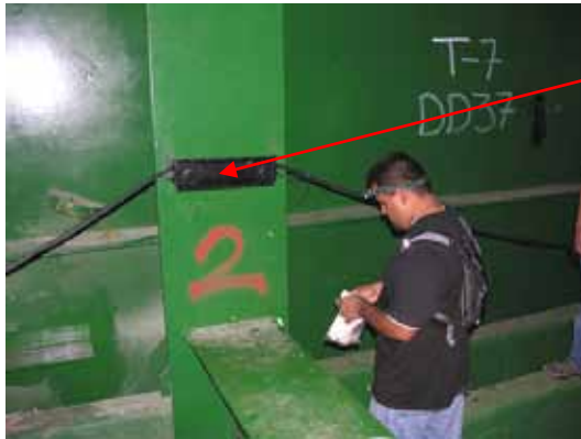
Splice tray for segment 2.
