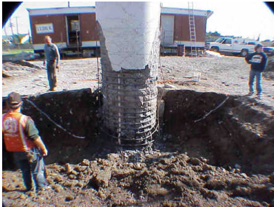
Figure 8. View of the stack after failure.
