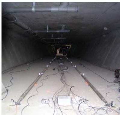
Fig. 5. FBG Bending Gauge layout inside the bridge girder
