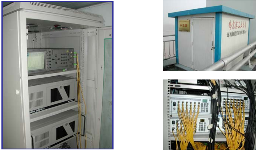
Figure 4 FBG sensor monitoring system
