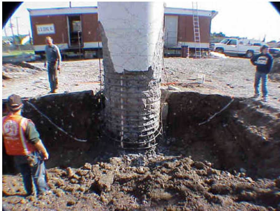
Figure 8. View of the stack after failure.
