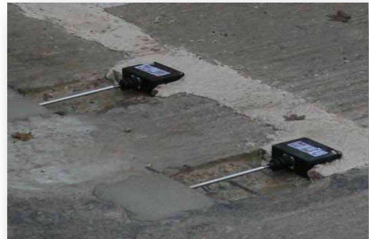
Close up of deck displacement sensors.
