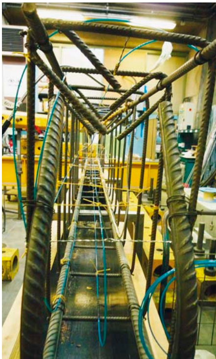
Figure 6: Reinforced concrete girder with fibre-optic cable (blue) before filling with concrete. The cable runs as a loop in the upper and lower segment to capture tensile and compression stresses (image source: [1])
